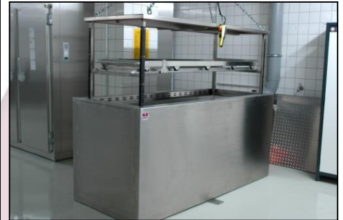
MA-1343.1 Preservation cuvette installed in an embalming room with explosion proof requirements
