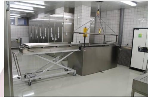
MA-1343.1 Loading / unloading procedure of a preservation cuvette in an embalming room
